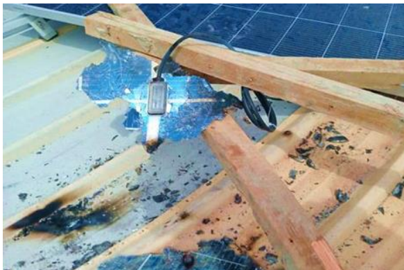
Figure 1: Junction box of the shattered solar panel that was ignited.
